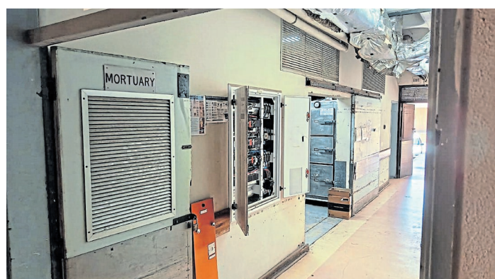
AT RISK: A state mortuary at Dora Nginza Hospital was allegedly affected by power failures this week, raising concerns about how bodies were being preserved. Picture: EUGENE COETZEE
